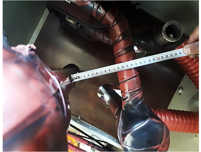
Fig. 3. Measured Phase to phase clearance (11 cm; Note that the Raychem strip insulator was wrapped on some parts of the busbar before the incident and did not have thickness more than 0.5 cm)
