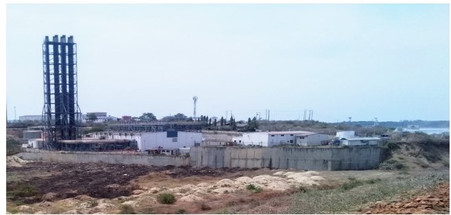
Fig. 1. Kipevu III 120 MW diesel engine power plant (Photo taken by 1st Author During Plant Construction).
