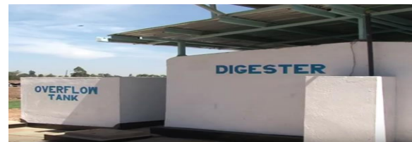
Fig. 5. Hydrolysis, digester, overflow, and treatment tanks (Photographed by researcher)
