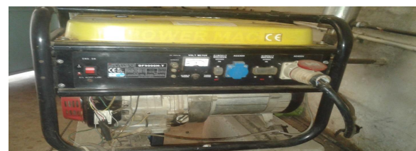
Fig. 6. Front view of the biogas generator at Nyongara slaughterhouse (photo by researchers)
