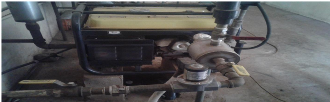
Fig. 7. Side view of the biogas engine unit at Nyongara slaughterhouse (photo by researchers)
