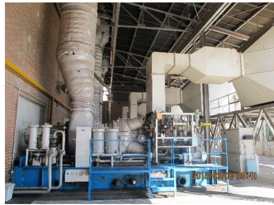
Fig. 1. A view of the station's turbines.
